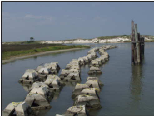
These breakwaters are protecting the Saw Grass Point Salt Marsh from erosion caused by wind and boat traffic in the area.
